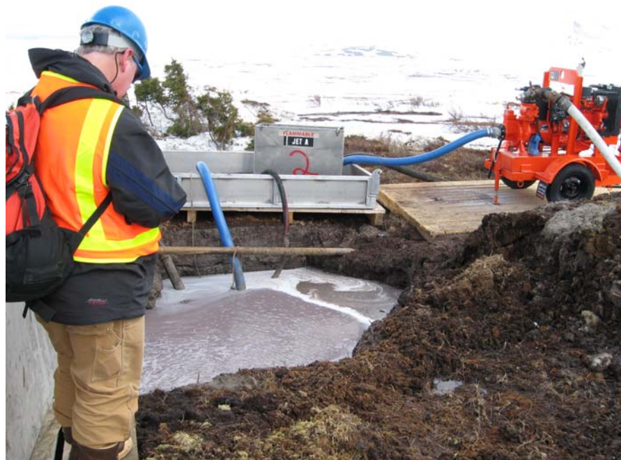
Figure 5. Drilling water sump, pump, and fuel storage at drill rig number 1. Drilling water was discharged onto uplands over 500 feet away from the drill rig through the white hose.
